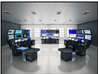
PLANT: BIG CREEK -Big Creek, CA OPERATOR: Southern California Edison Year: 2013 Product Line: Talon-2
